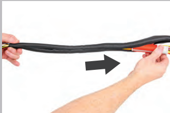
4. Hold cable and wrap together at one end and pull tool down along cable bundle.
